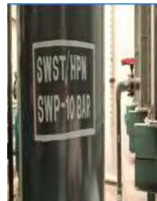
SWP labelling of all pressure vessels
