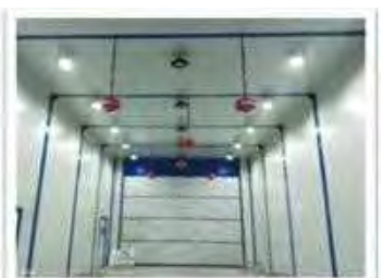
Modular Fire fighting arrangements in Paint Booth
