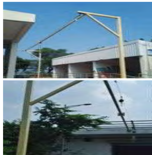
Implemented lifeline system in Scrap Yard, WMS Scrap, LG Dock, and OCM Dock.
