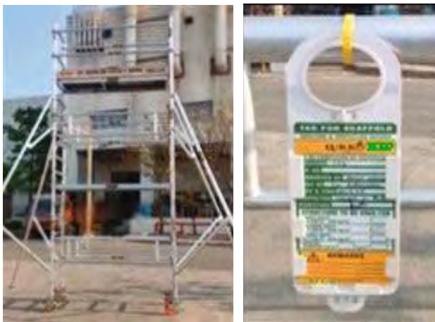
CEHS Approved Standard Scaffolding with Safety Tags with Trained and certified Scaffolding erector (30) and Inspector (4)
