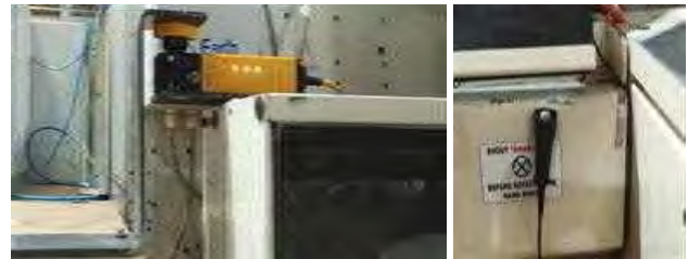
GDX : Dead man's Switch | RFID – Coded safety Interlocks prevent override | control supervision are maintained during
