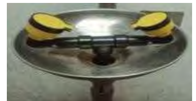
All eyewash station provided with dust flaps to prevent clogging of nozzles
