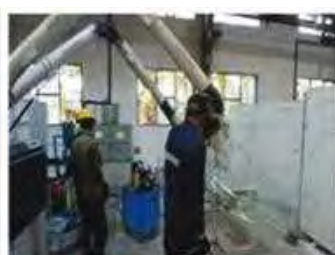
Fume extractor implementation in welding area
