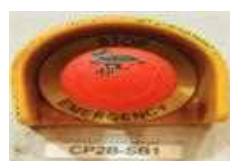
All Emergency stop switch with proper labelling done
