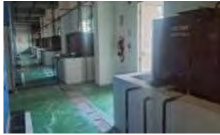
Day tank Dyke Volume increase to contain all spillage in case of failure
