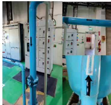
All pipelines provided with Directional arrows.
