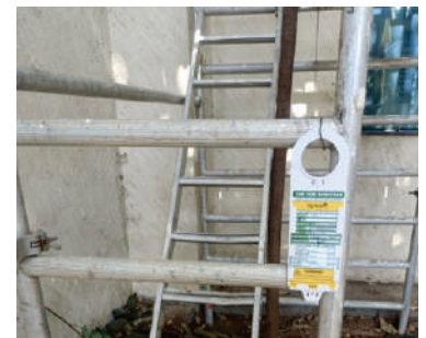
System of Inspection and tagging of Scaffolds for safe Use.
