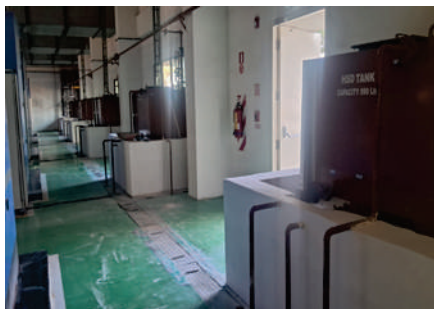
Day tank Dyke Volume increase to contain all spillage in case of failure
