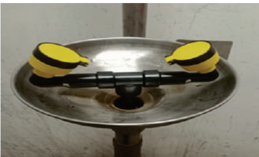
All eyewash station provided with dust flaps to prevent clogging of nozzles
