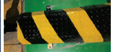
All area with pipelines above floor covered with flat surface and hazard marking done.
