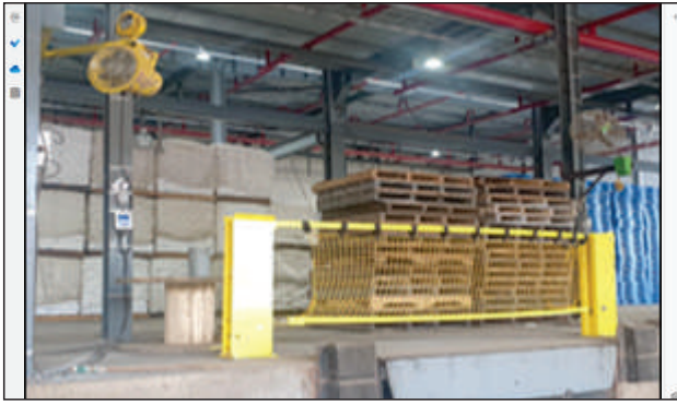
Dock Impact Barrier Air Blower & Spotlight Provision
