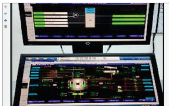
Interlock inbuilt in DCS
