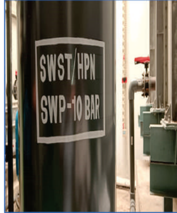
SWP labelling of all pressure vessels
