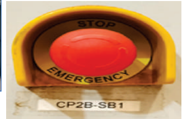
All Emergency stop switch with proper labelling done
