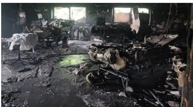
Charred remains of the ICU at Shrey Hospital in Ahmedabad, Gujarat.
