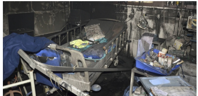
Charred remains of the ICU at Uday Shivanand Hospital in Rajkot, Gujarat.
