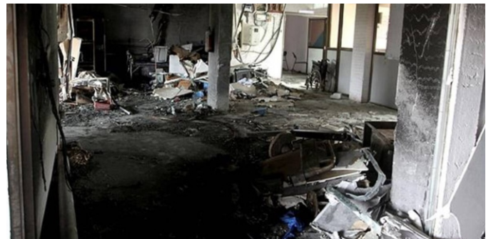
Remains of the ICU of The Patel Welfare Hospital in Bharuch.
